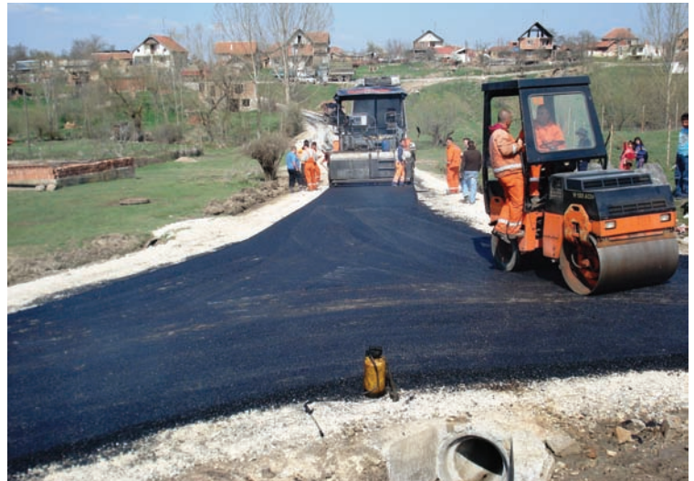
Mercy Corps Kosovo, MISI Program road asphalting project in the village of Gracë/Grace, Vushtri/Vucitrn.
